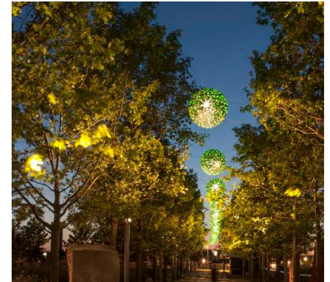
Claremont Park - Lighting installations
